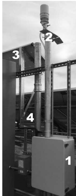
Figure 2: SolarSCADA Typical Install
