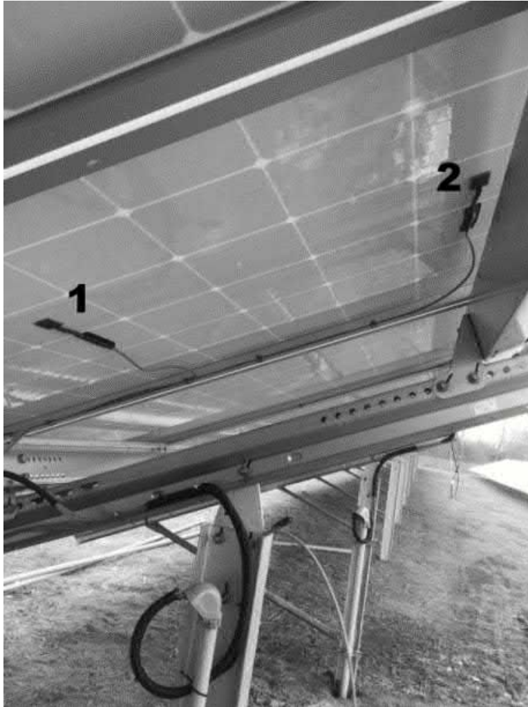
Figure 6: Properly Installed Back of Module (BOM) Temperature Sensors
